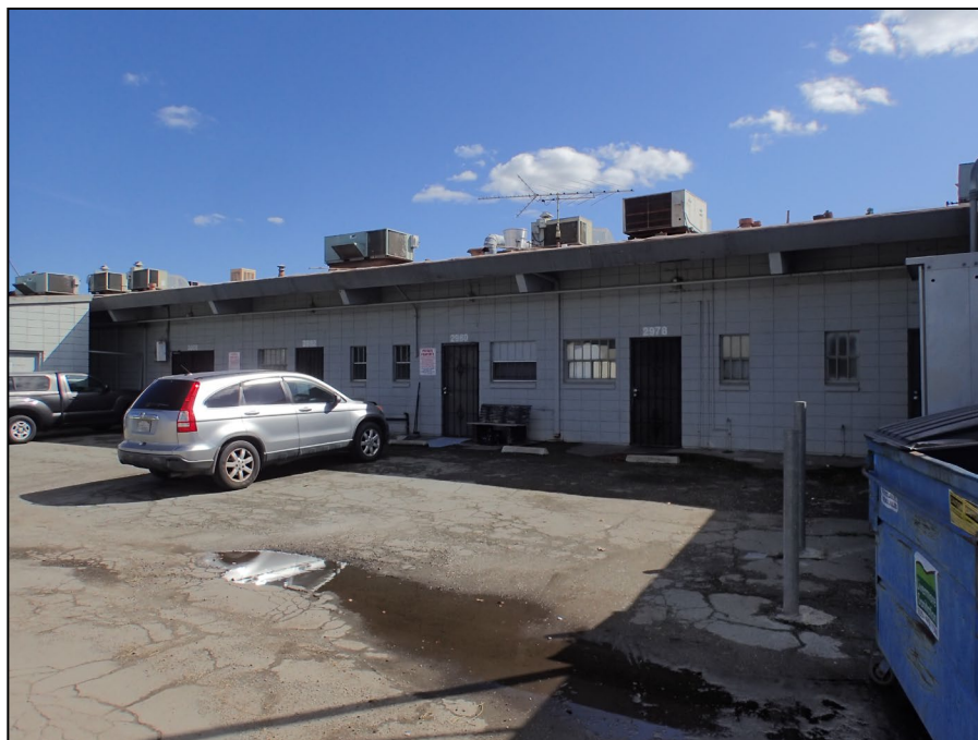
Vineyard Shopping Center. Primary building. Anchor tenant space, north (rear) façade. View southeast. LSA photograph 3/18/25.
