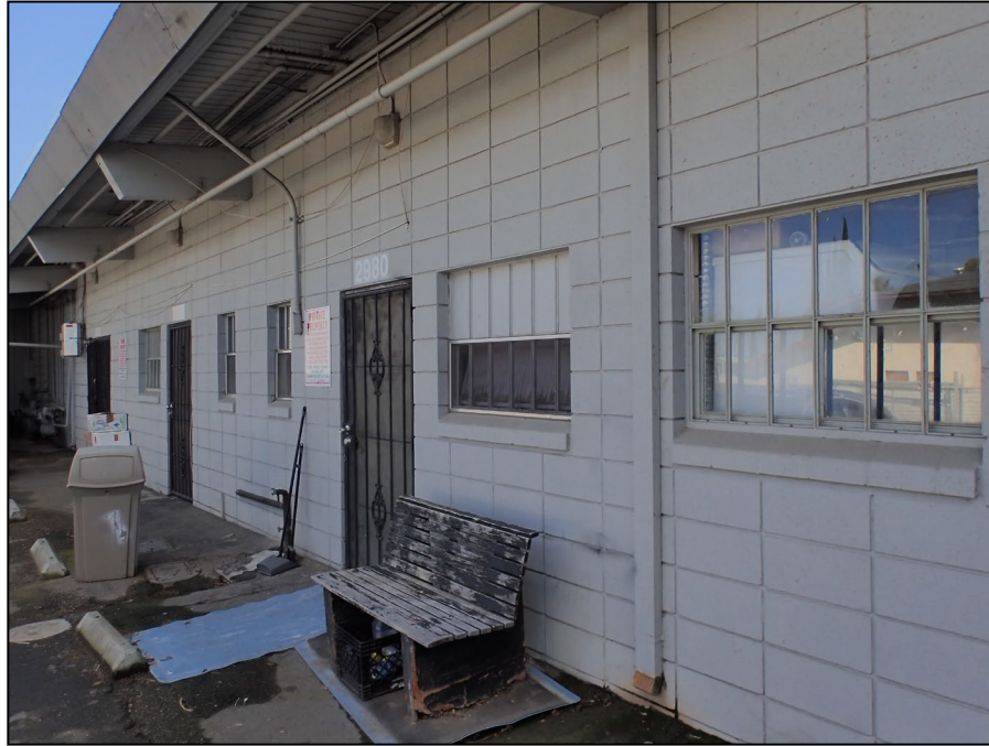
Vineyard Shopping Center. Primary building. Anchor tenant space, north (rear) façade. View east. LSA photograph 3/18/25.
