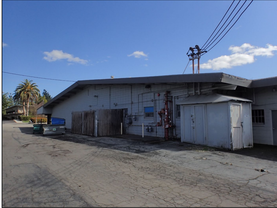
Vineyard Shopping Center. Primary building. Anchor tenant space, north (rear) façade. View southeast. LSA photograph 3/18/25.
