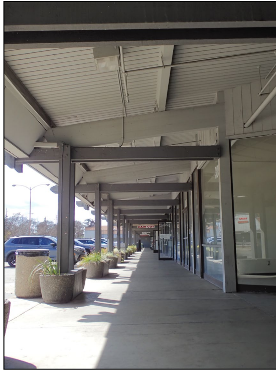
Vineyard Shopping Center. Primary building. Covered walkway along tenant space entrances. View west. LSA photograph 3/18/25.
