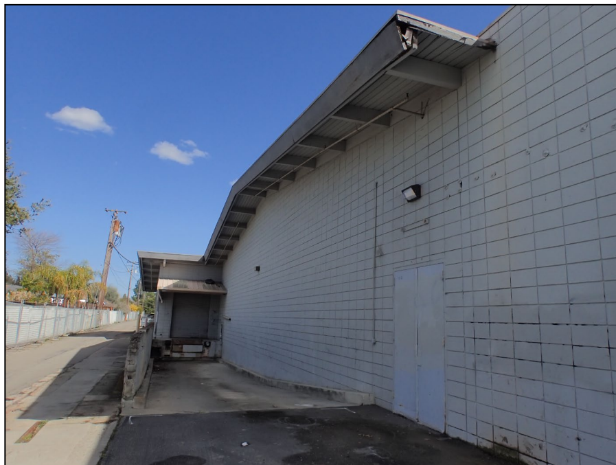
Vineyard Shopping Center. Primary building. Western anchor tenant space, north (rear) façade. Loading ramp, dock, and roof eave. View east. LSA photograph 3/18/25.
